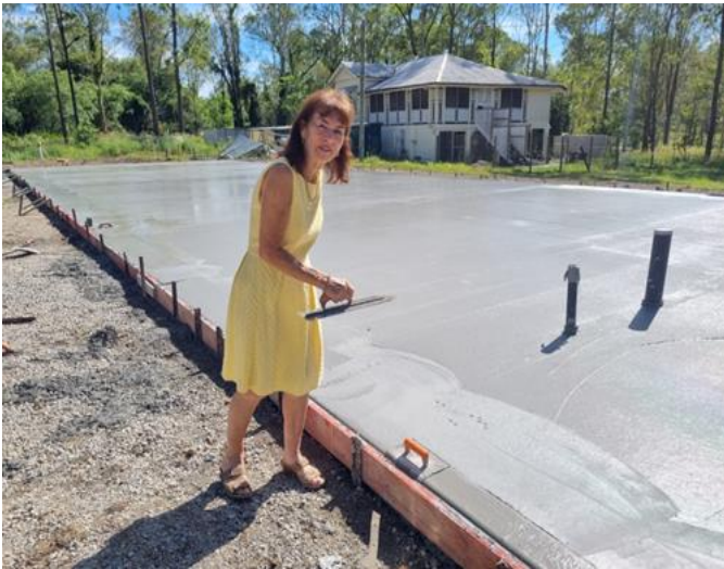
ATAC Board Chair Ms. Irene Bayldon trying her skills on the concrete slab. Irene has been supporting the project and wants it to be fully completed as soon as possible.
