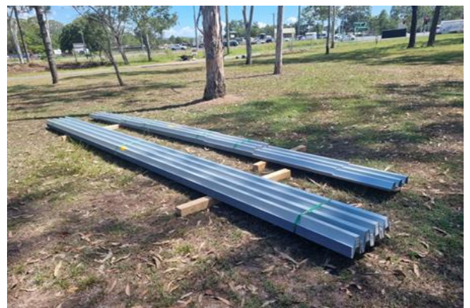
Shed material arriving for the construction to start as soon as possible.
