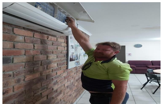
Daniel Springall (Parent) servicing ATAC air conditioners for free. Big thank you Dan from the ATAC Board, staff, and students. It would make a great difference to maintain temperatures in our classroom and admin building. Thanks for Keeping us warm.
