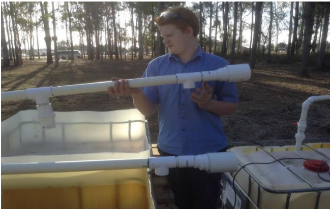
Nick Springall the leader of the Aquaponics project setting up the piping system
