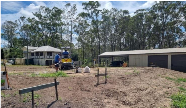
The raised pad level to meet the Logan City Council flood levels. The shed project was delayed for two years due previous contractor error. What a great relief.
