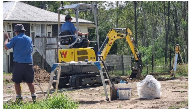
The excavator of new contractor digging trenches for plumbing works. Weather is holding and we expect concrete pads to be completed by next week.
